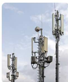
Signal base station
